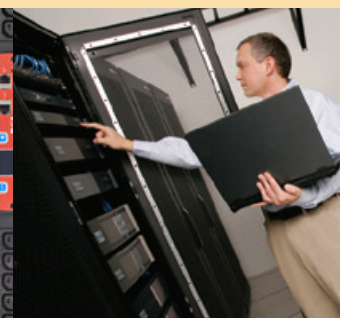
Enclosures with rackmount UPSs
