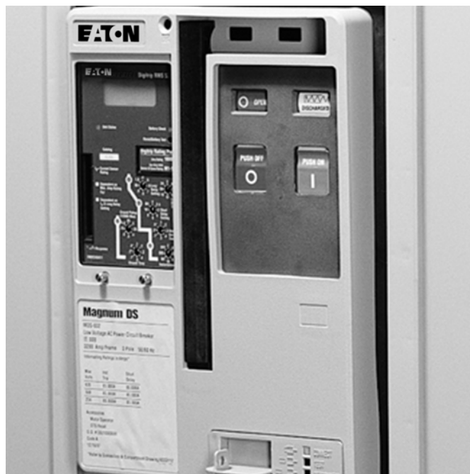
Through-the-Door Design for Human Interface with the Breaker Compartment Door Closed
