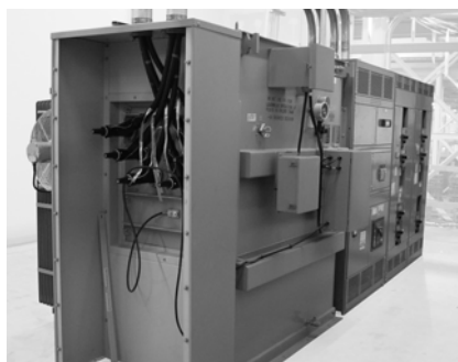
VFI with Secondary Unit Substation
