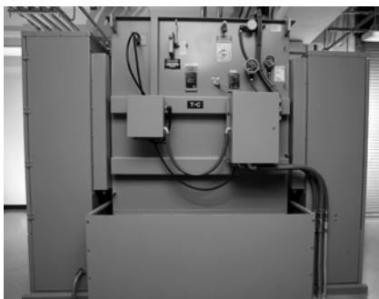
VFI Primary with Secondary Cable Connections and Containment Pan
