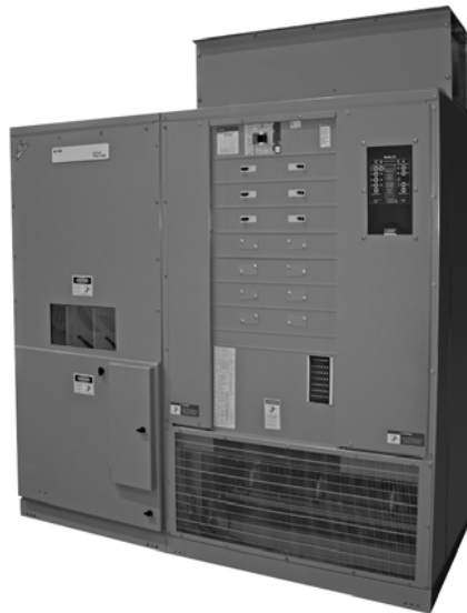
Unitized Power Center
