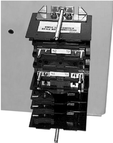
Test Block with Cover Removed
