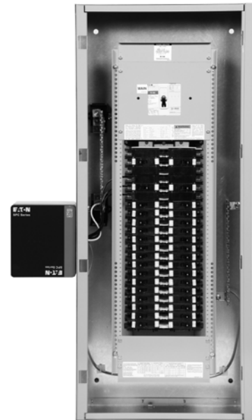
SPC Device Mounted to an Eaton Panelboard
