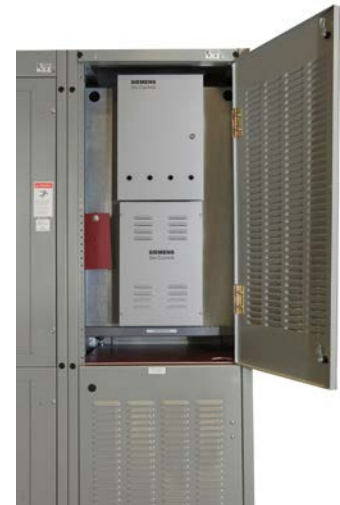
Building Management System
