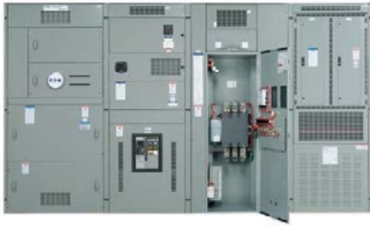
Integrated Facility System Switchboards
