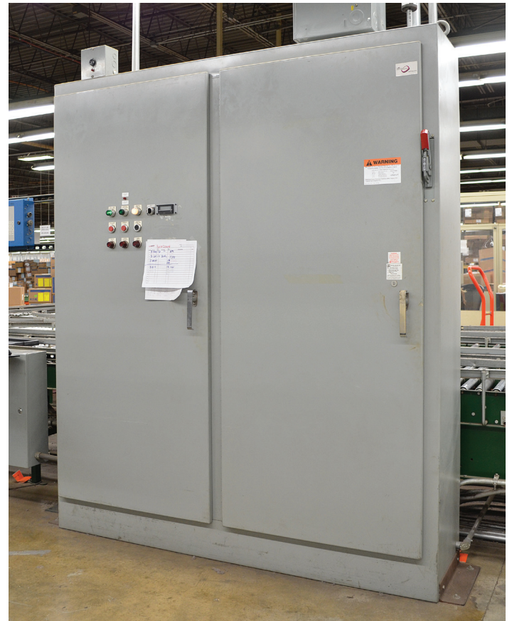
Manufacturer’s nameplate with equipment SCCR marking appears on the enclosure’s interior.
