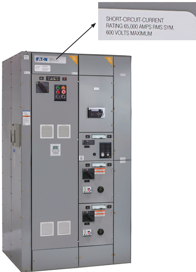
Manufacturer's nameplate with equipment SCCR marking.
