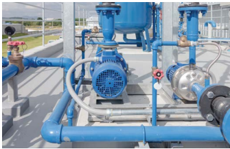
Pumps and compressors
